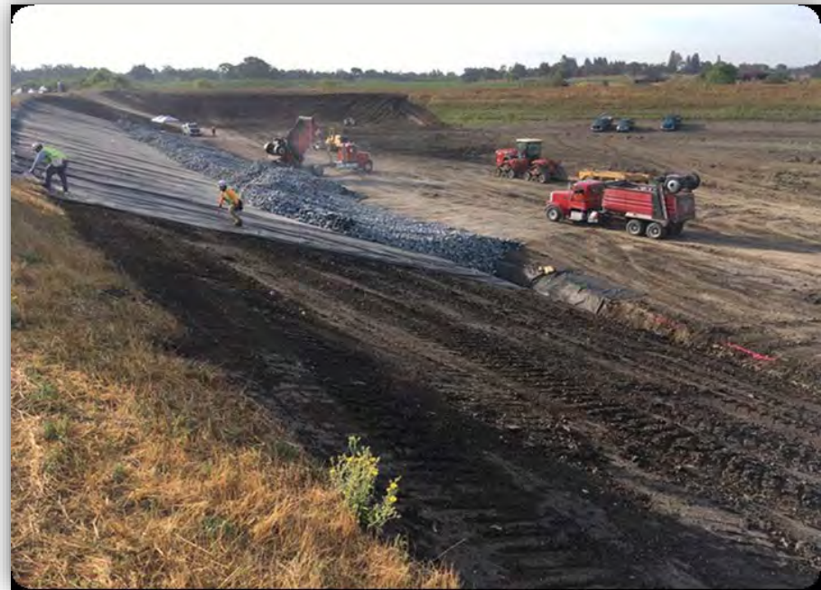
Northerly Slope Protection Delta Pond
